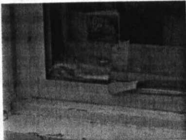
Duct tape used to repair window.
