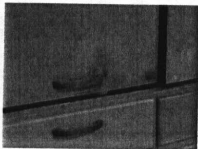
Deteriorating cabinets in original portion of building.
