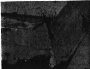
Badly bent metal flashing.
