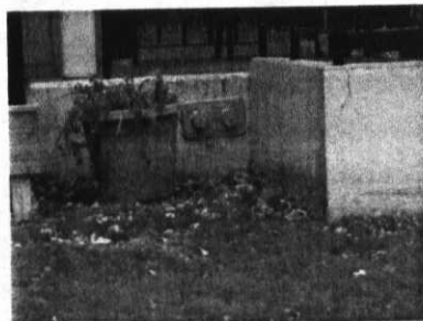
Limited access to fire department siamese connection.
