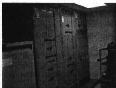
Switchboard and distribution panels.
