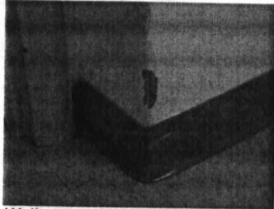
Wall corner damage.
