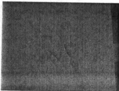
Paint peeling from wall in Library.
