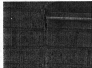
Deterioration of expansion joint.
