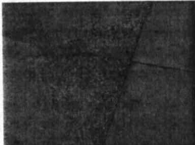
Spalling concrete paving. Note pop-outs.
