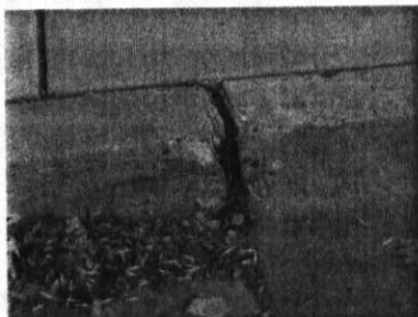
Damaged concrete curb.
