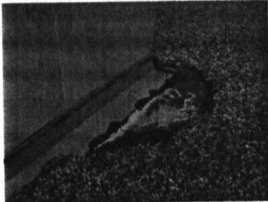
Aggregate surfacing shifting.
