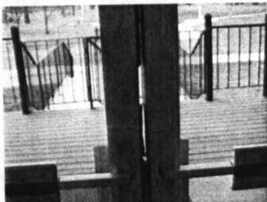
Lack of weatherstripping between door leafs.
