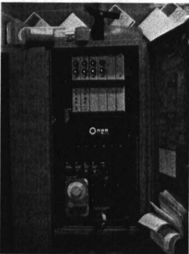
Transfer switch at Onan generator.
