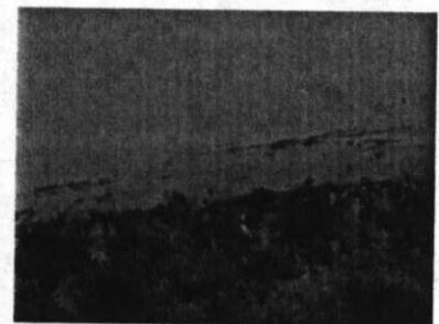
Paint damaged by lawn care equipment.
