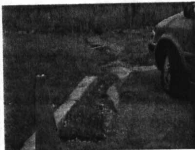
Erosion at staff parking lot.
