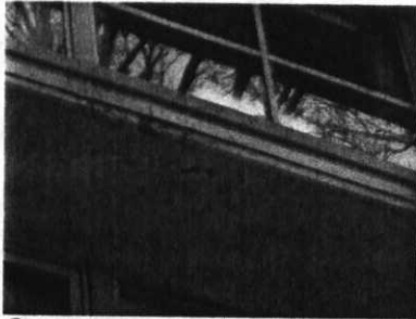
Concrete sun shade spalling.
