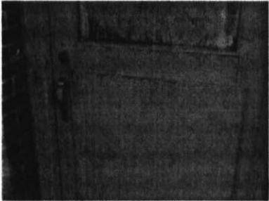
Deteriorating finish and wood.
