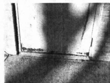
Deteriorating finish and rusting door.
