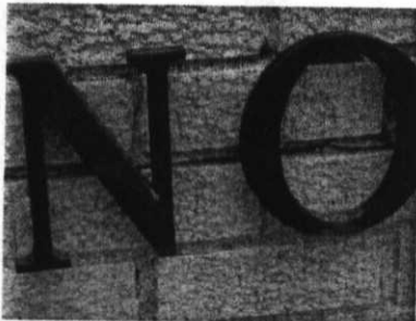
Deteriorating mortar joints.
