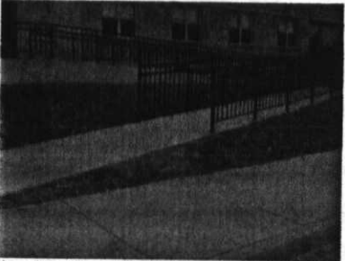
Lack of handrail extensions at ramp.
