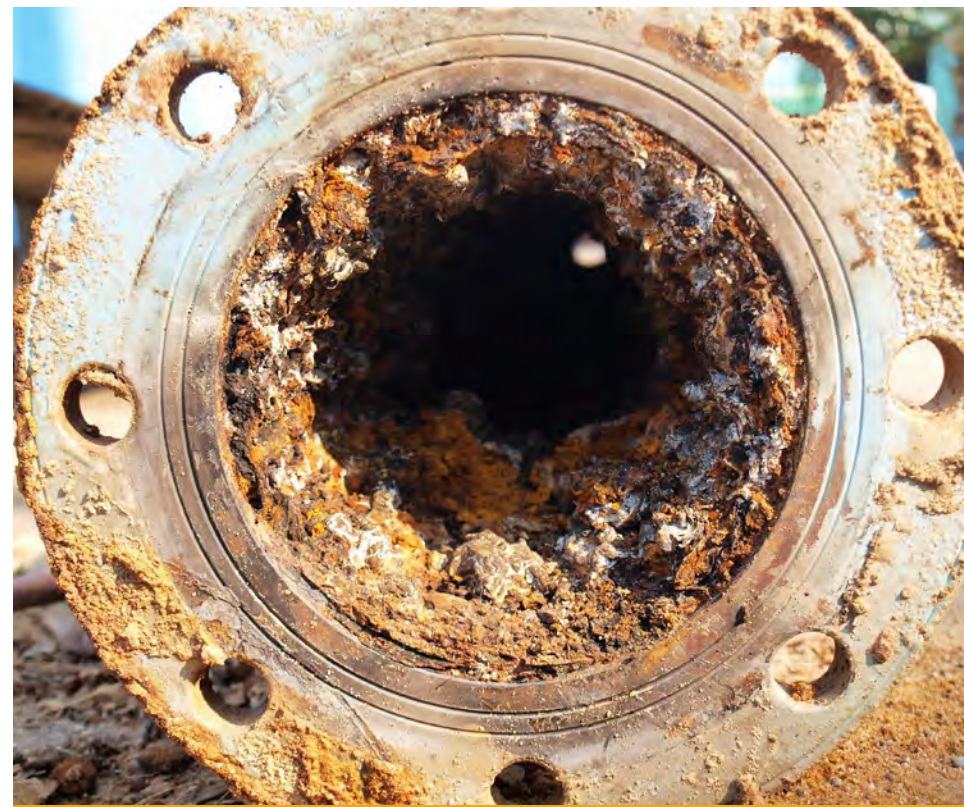
A new sanitary sewer line will prevent inflow and infiltration, saving in maintenance costs.
