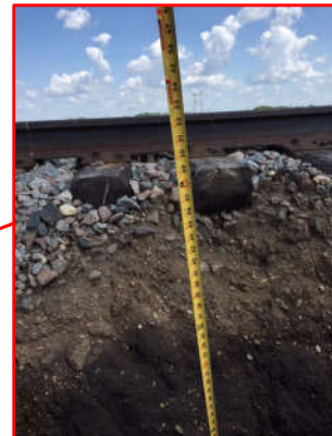
Shows depth of hole created by collapsed drainage culvert.
