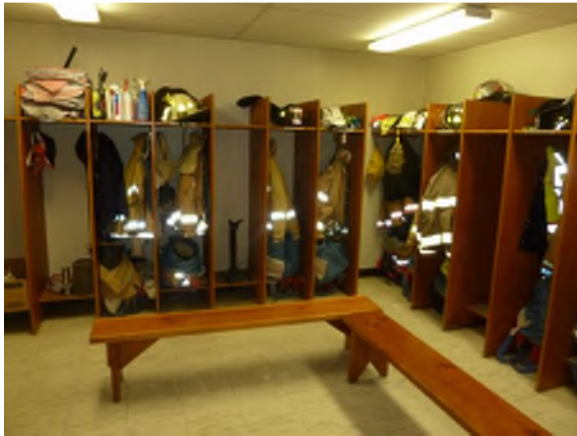
Solid panels at gear lockers restrict evaporative drying of turnout gear
