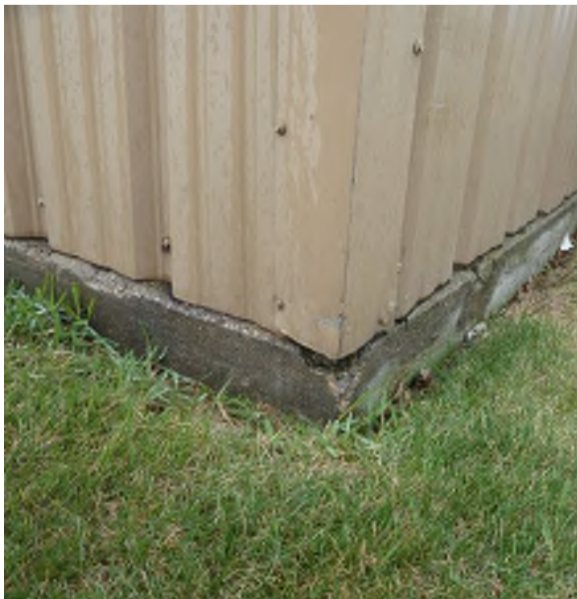
Spalling at concrete footing wall at northeast corner of building
