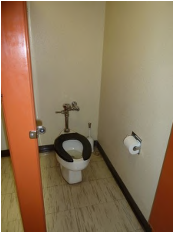
Lavatory, shower, urinal, and toilet not accessible
