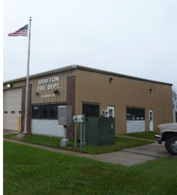
Electrical equipment not protected from vehicle traffic by bollards
