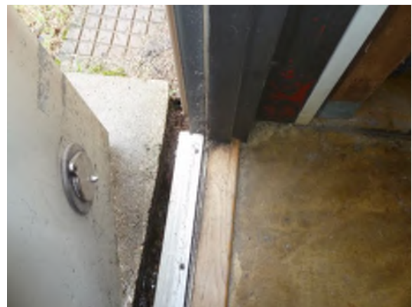
Rear door stoop has separated from building
