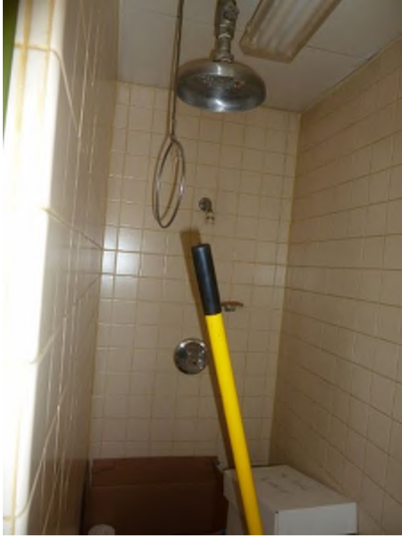
Shower needs re-grouting and new curtain
