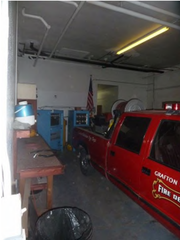
No exhaust removal system in maintenance bay
