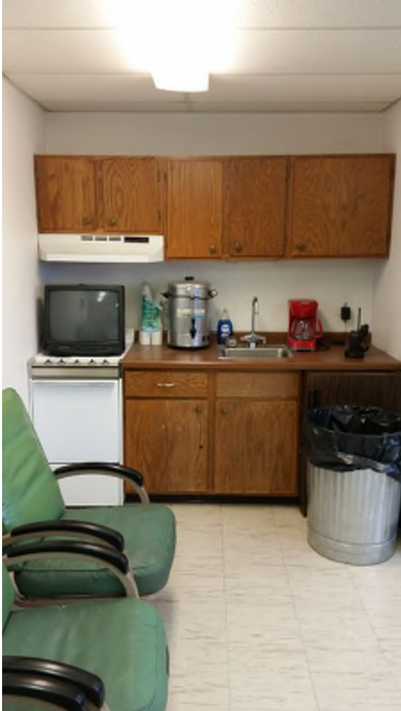
Stove and cabinets at end of useful service life
