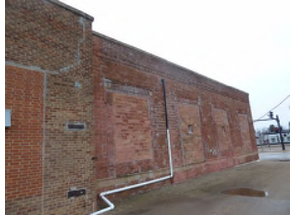
Exterior needs tuck pointing along the north wall
