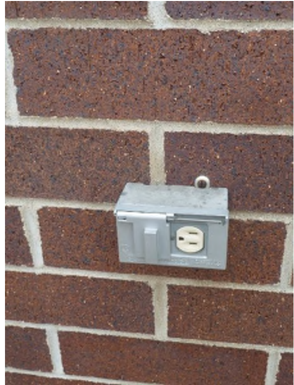
Exterior electrical outlet missing weather protection cover
