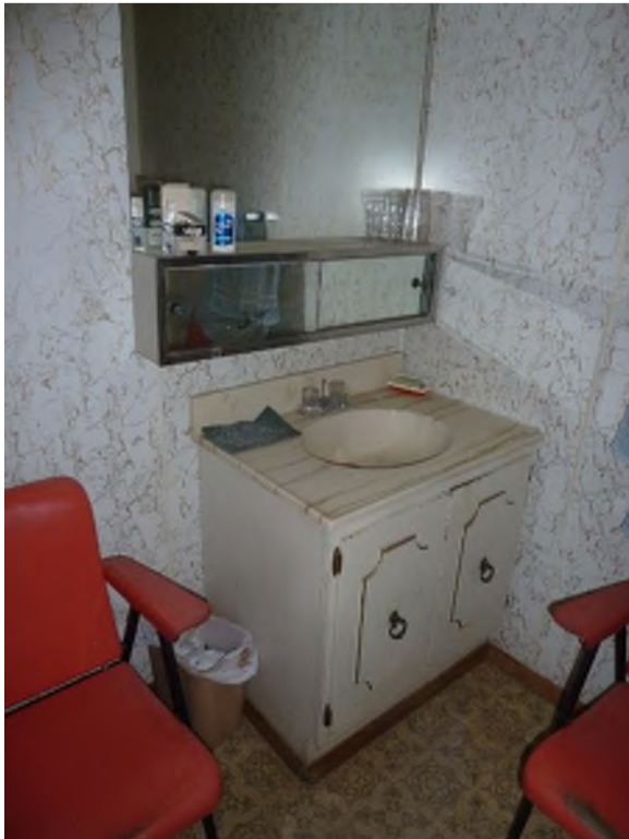
Fixtures and finishes in toilet room past the end of their useful life
