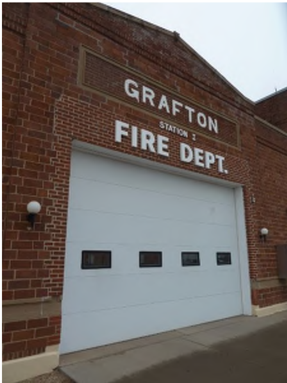
Apparatus door jambs need to be re-caulked
