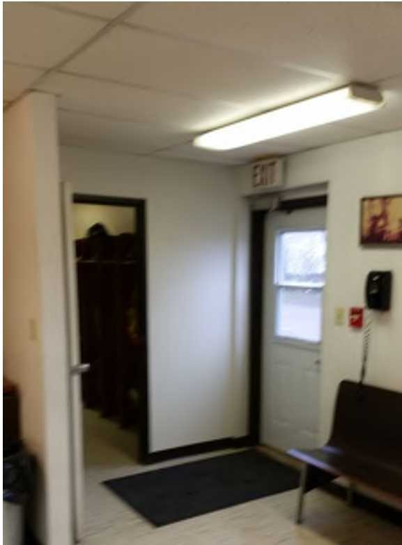
Exit lights are not operational throughout the facility
