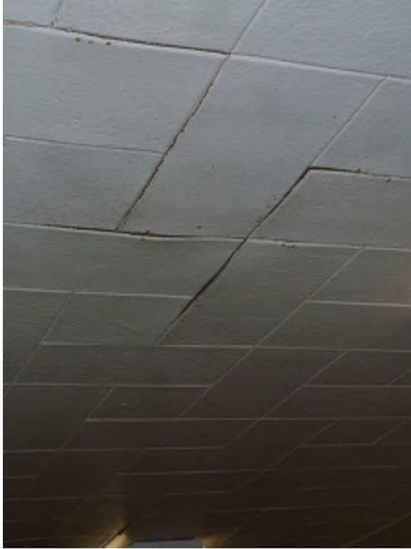
Ceiling tiles loose at Firemen's Hall
