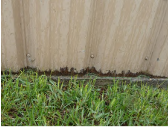
Bottom of metal wall panels beginning to deteriorate
