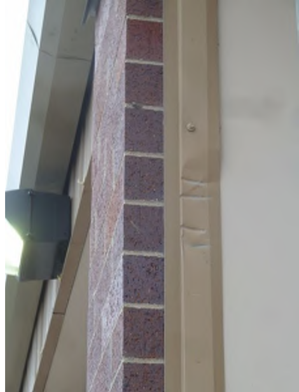
The west side of apparatus door closest to the office is damaged
