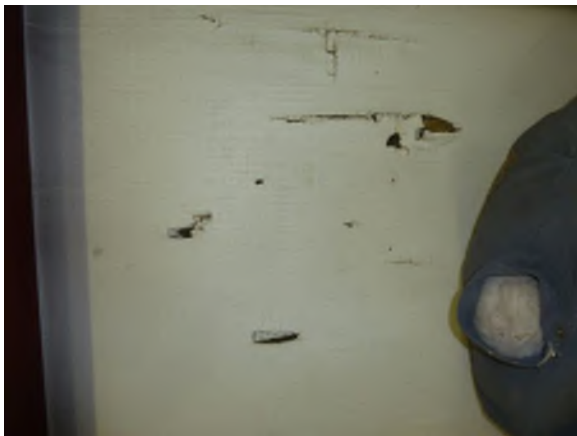
Frequent tears in vapor barrier at ceiling/walls throughout facility allows moisture into batt insulation, rendering it much less efficient at resisting heat transfer
