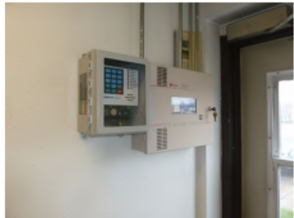
Fire alarm panel is protruding object
