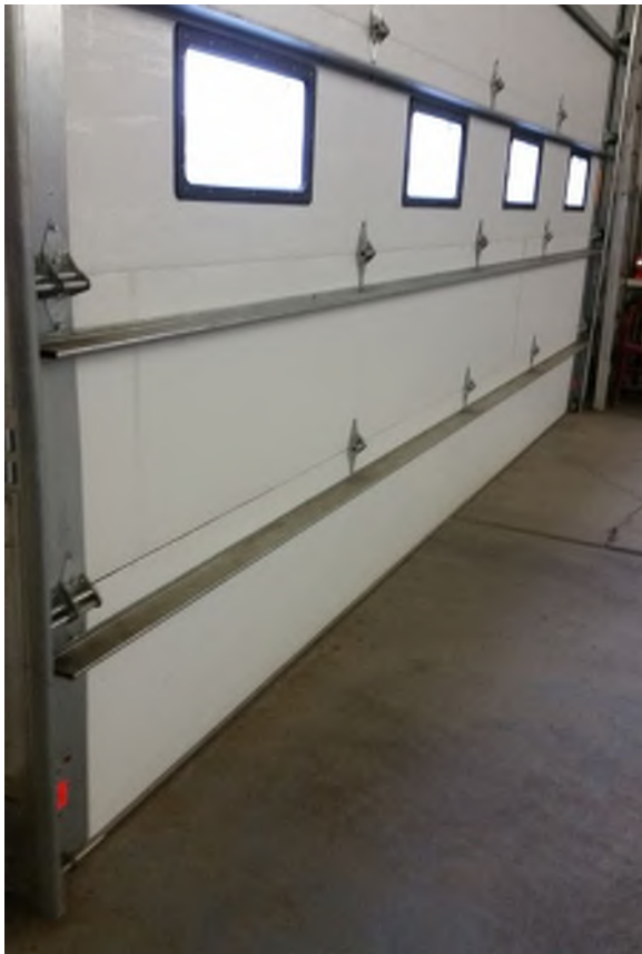
No photo-eyes on bay doors, creating pinning/ crushing hazard
