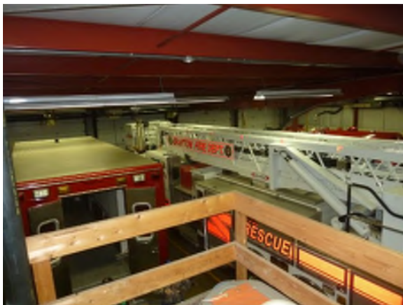
No sprinkler system
