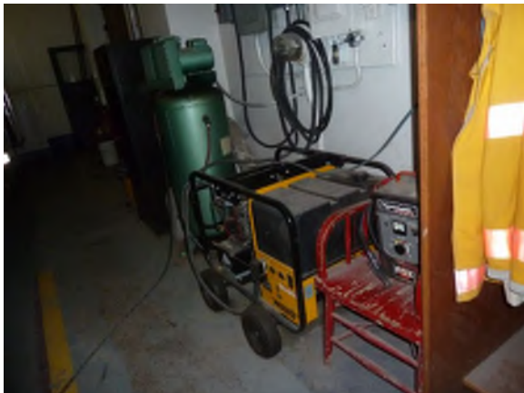
Equipment stored in front of electrical panels
