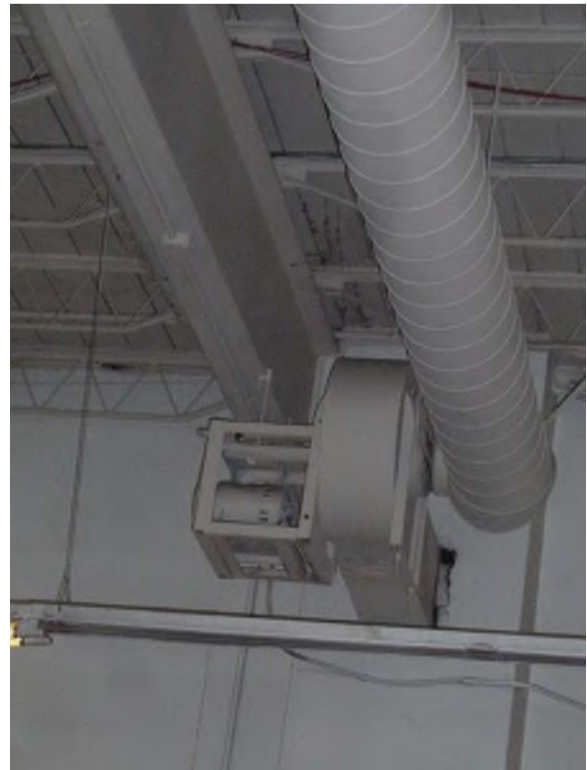
Mechanical exhaust system motor needs maintenance
