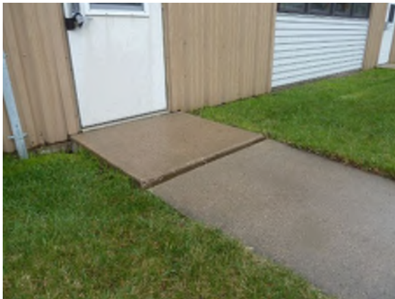
Sidewalks heaving/ settling compared to stoops, creating trip hazard
