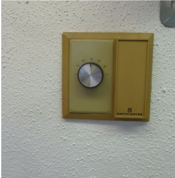
Client reports that in-floor radiant heat system broken
