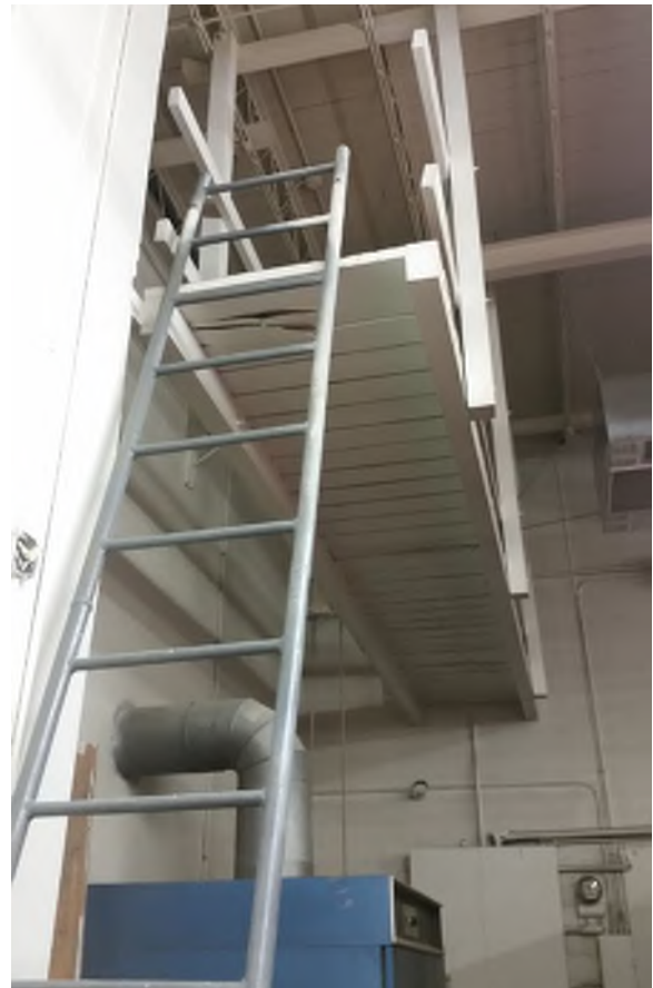
Ladder to hose drying not secured
