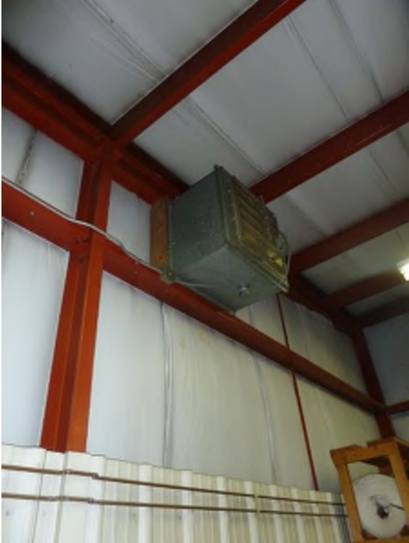
Exhaust fan needs maintenance, rebalancing
