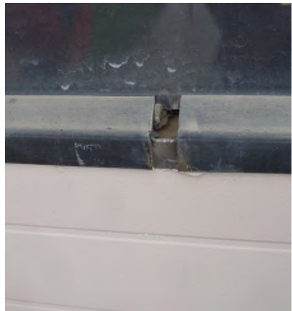
Glazing panels in sectional overhead doors have large gaps at seals
