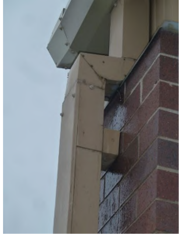
Southwest downspout damaged and leaking down face of building
