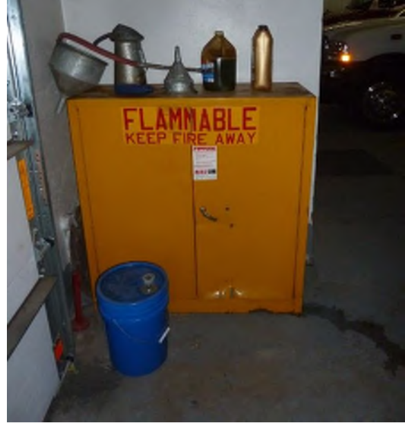
Flammable cabinet bent, no longer able to contain fumes
