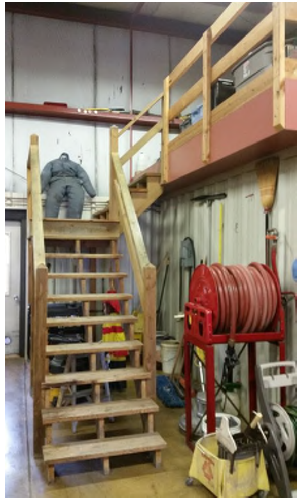
Staircase has open risers and non-compliant handrails/ guardrails
