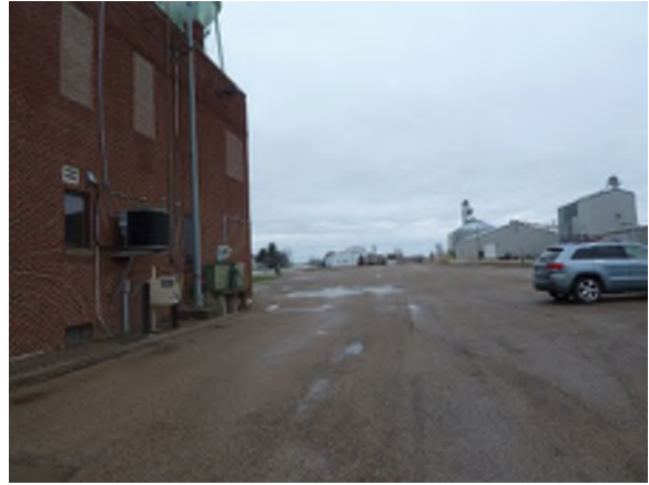
Asphalt past the end of its useful service life. Exhibiting potholes, cracks, disintegrating top layer
