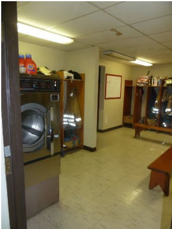
Evidence of roof leaks at ceiling tiles. Client reports having repaired roof several times.
