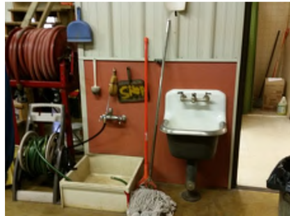
Insufficient decontamination space for SBCA masks and equipment
