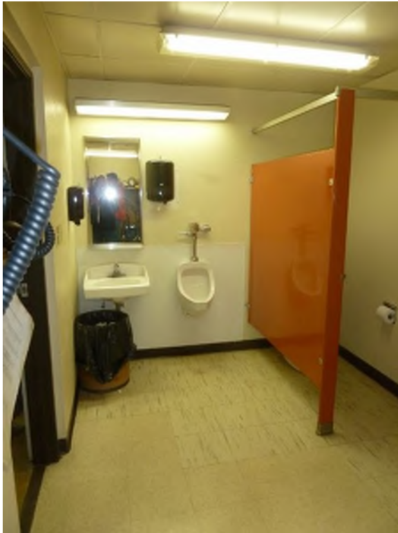
No separate locker and toilet facilities for females
