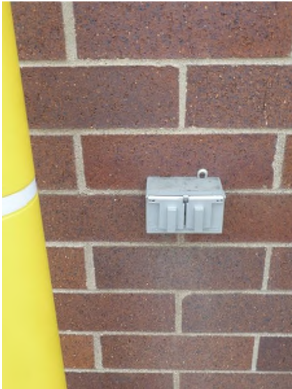
Exterior electrical outlets do not comply with current Electrical Code
