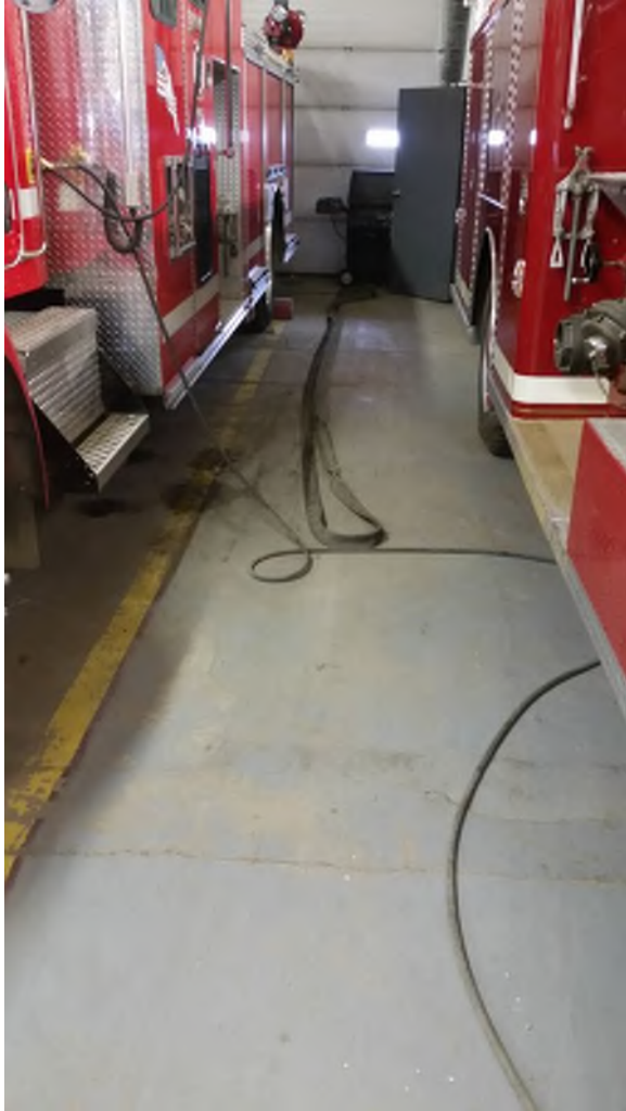
Shore lines laying on floor create tripping hazard
