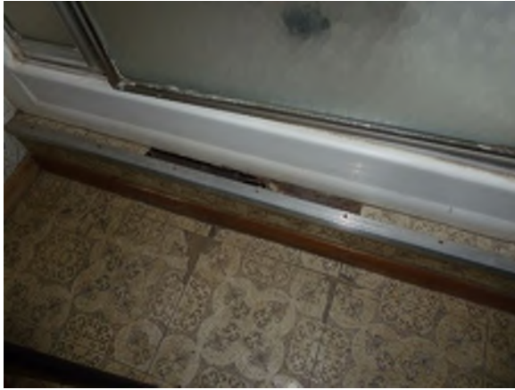
Wood framing below shower pan not protected from moisture and shows evidence of disintegration
