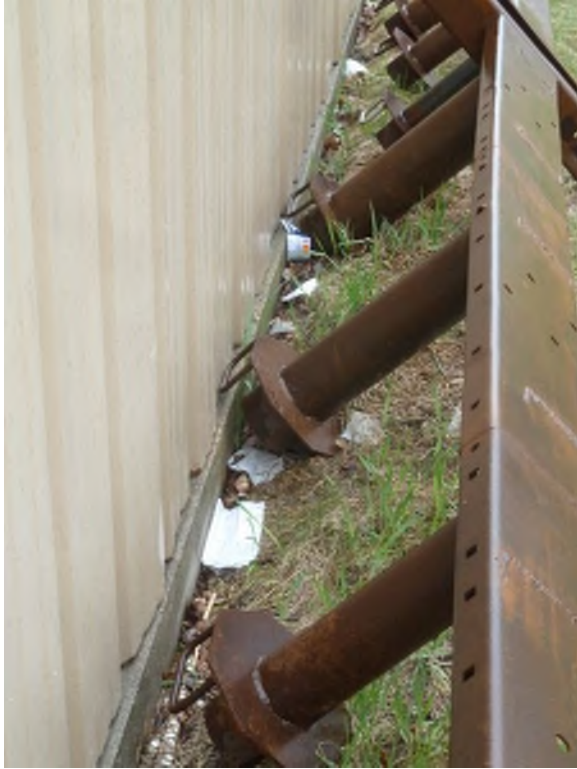
Grade slopes towards footing at north wall
