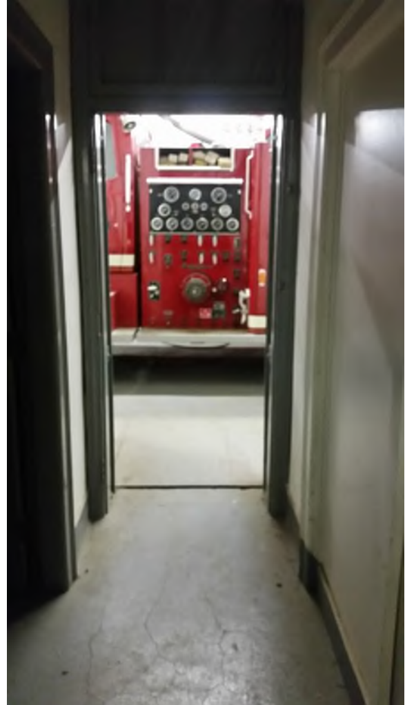
No wheelchair maneuvering clearance at the doors to/ from corridor
