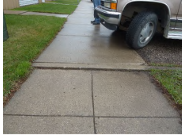
No detectible warning features between sidewalk and parking spaces
