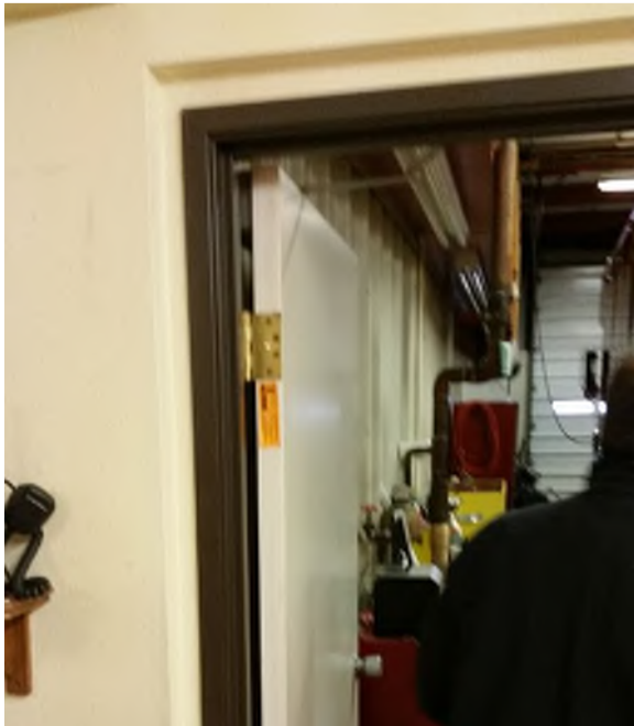
Fire rated doors held open by door stops
