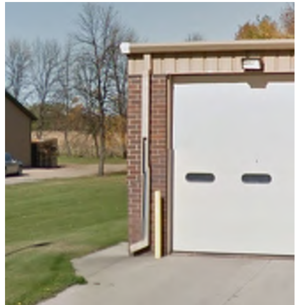
Southwest downspout discharges across sidewalk, creating potential for ice formation
