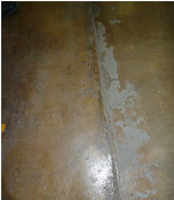
Concrete floor in apparatus bay showing signs of deterioration
