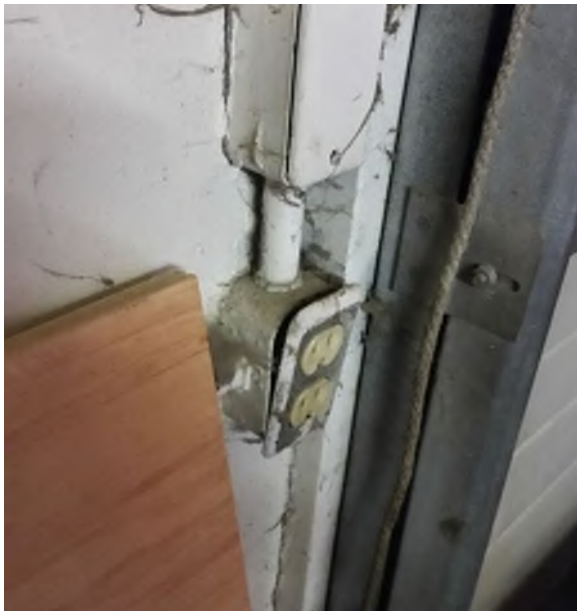
Unseated electrical cover plates
