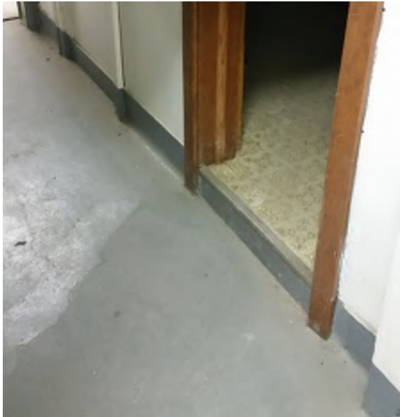
Toilet room not accessible due to step
