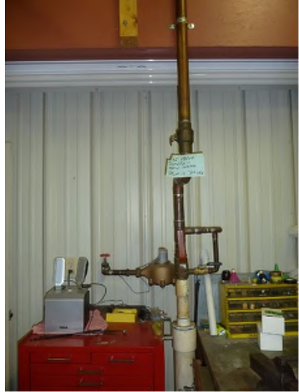
Water valve broken at street, creates water hammer problems inside building
