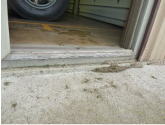
Exterior stoop at west side not flush with interior floor slab
