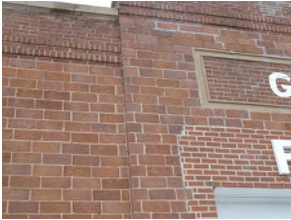
Exterior needs tuck pointing at parapet above the bay doors
