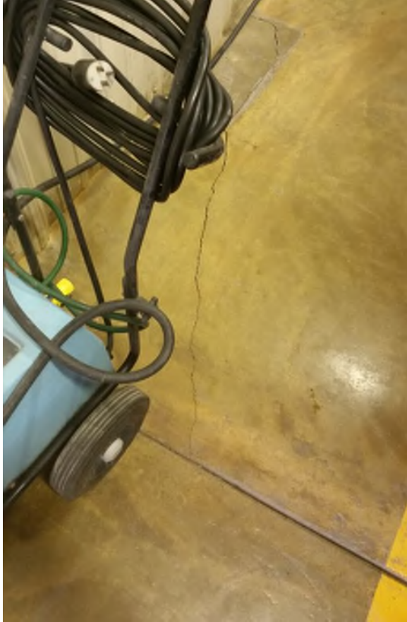
Concrete has cracked and settled in apparatus bays, creating trip hazard at joints
