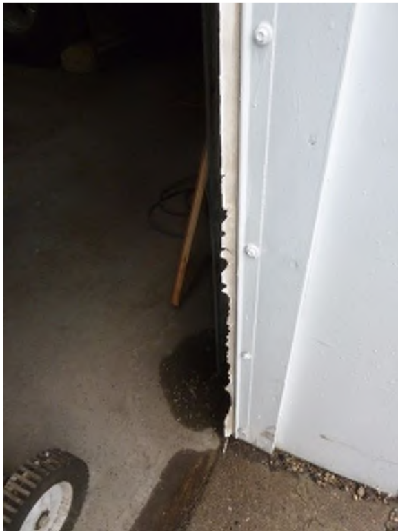
Weatherstripping at rear apparatus door needs replacement
