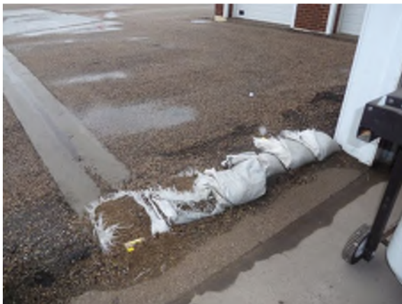
Grading at rear apparatus door slopes towards building
