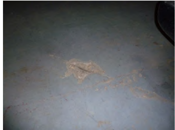
Cracks in floor, some down to rebar
