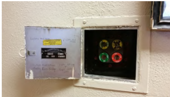
Fuse box serving Firemen's Hall no longer code compliant
