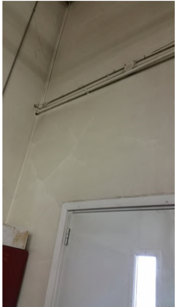
Plaster cracking and falling off interior walls
