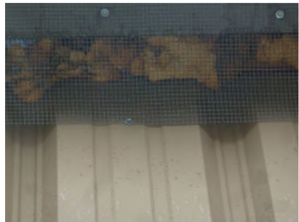
Spray foam insulation exposed on exterior
