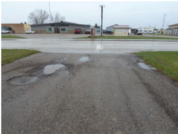
Asphalt at parking lot past the end of its useful service life. Exhibiting potholes, cracks, disintegrating top layer
