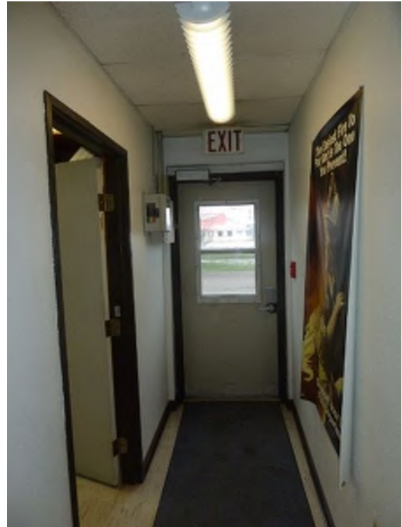
No wheelchair maneuvering clearance at the four doors to/ from corridor
