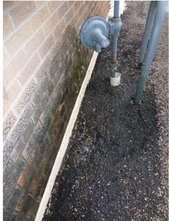
Roof drain discharges water at building wall, creating environment for molds and lichen and causing brick to spall and deteriorate
