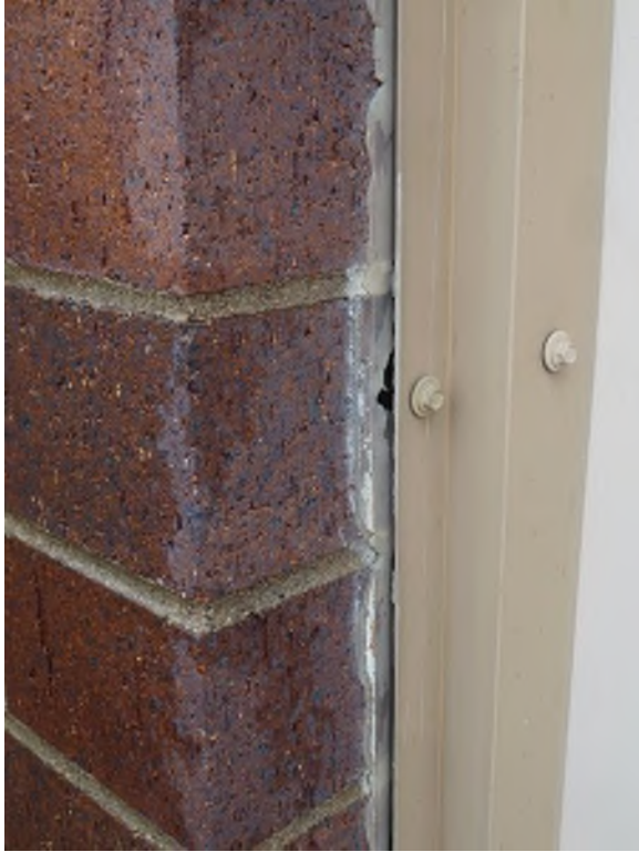
Sealant failing at all locations – needs to be re-caulked
