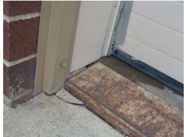
Weatherstripping at overhead doors damaged and needs replacement
