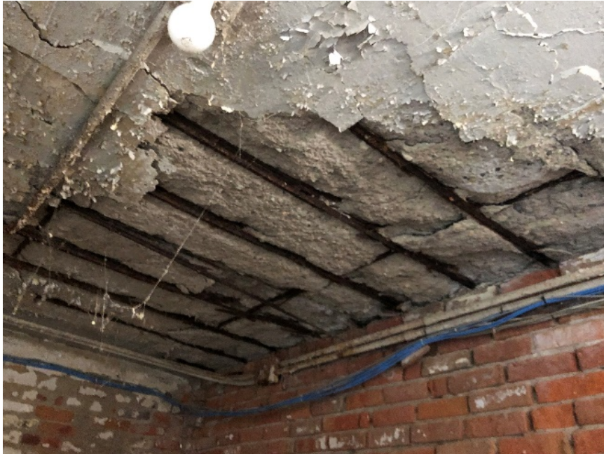
Image 8: Exposed Rebar in Basement
