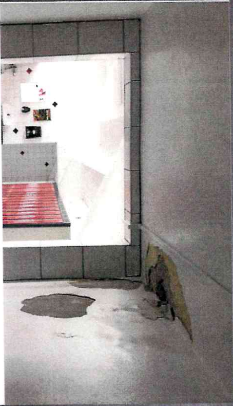
Water damage on ceiling and wall in boy's locker room
