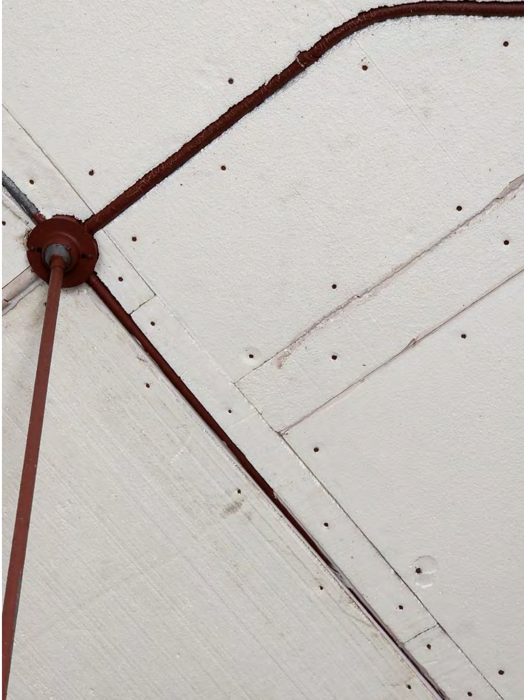
Nonstandard ceiling material. Electrical conduit showing signs of water damage and rusting. Lighting has not been upgraded. (Photo: 20240216_142219)
