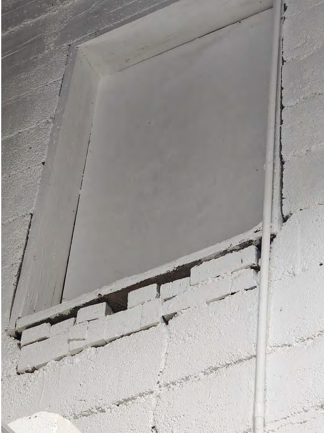
Window jambs and sills in poor condition and non-standard construction methods. Location of water and pest infiltration. (Photo: 20240411_135835)
