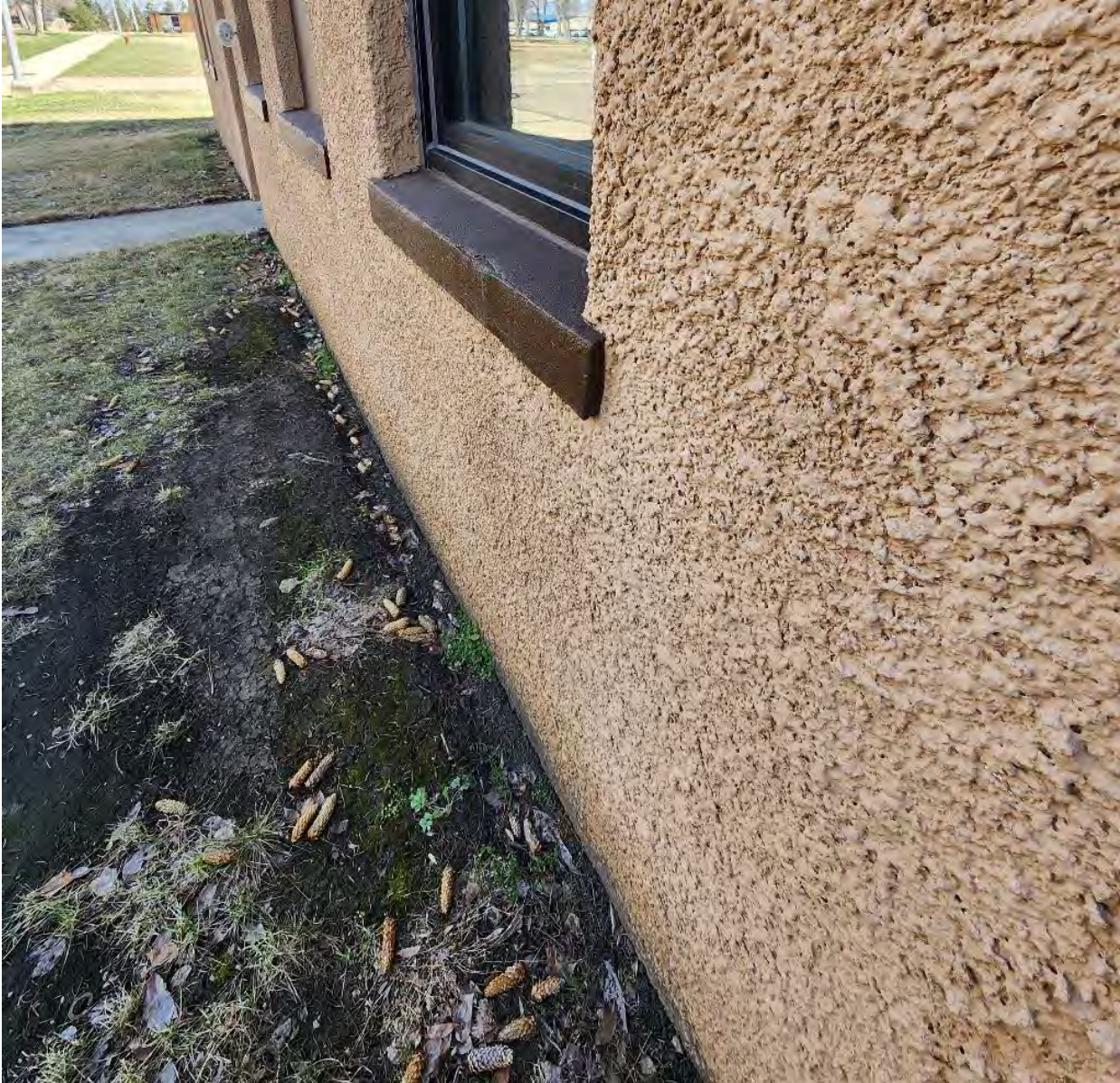
Exterior drainage along the wall and foundation in poor condition. Evidence of water sitting along the foundation wall. (Photo: 20240411_145949)
