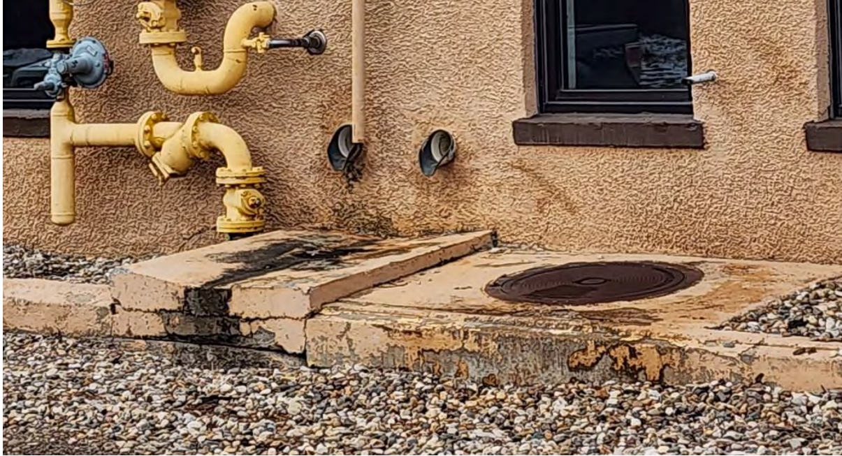
Exterior drainage along wall and foundation in poor condition. Evidence of water infiltration. (Photo: 20240216_1440009)
