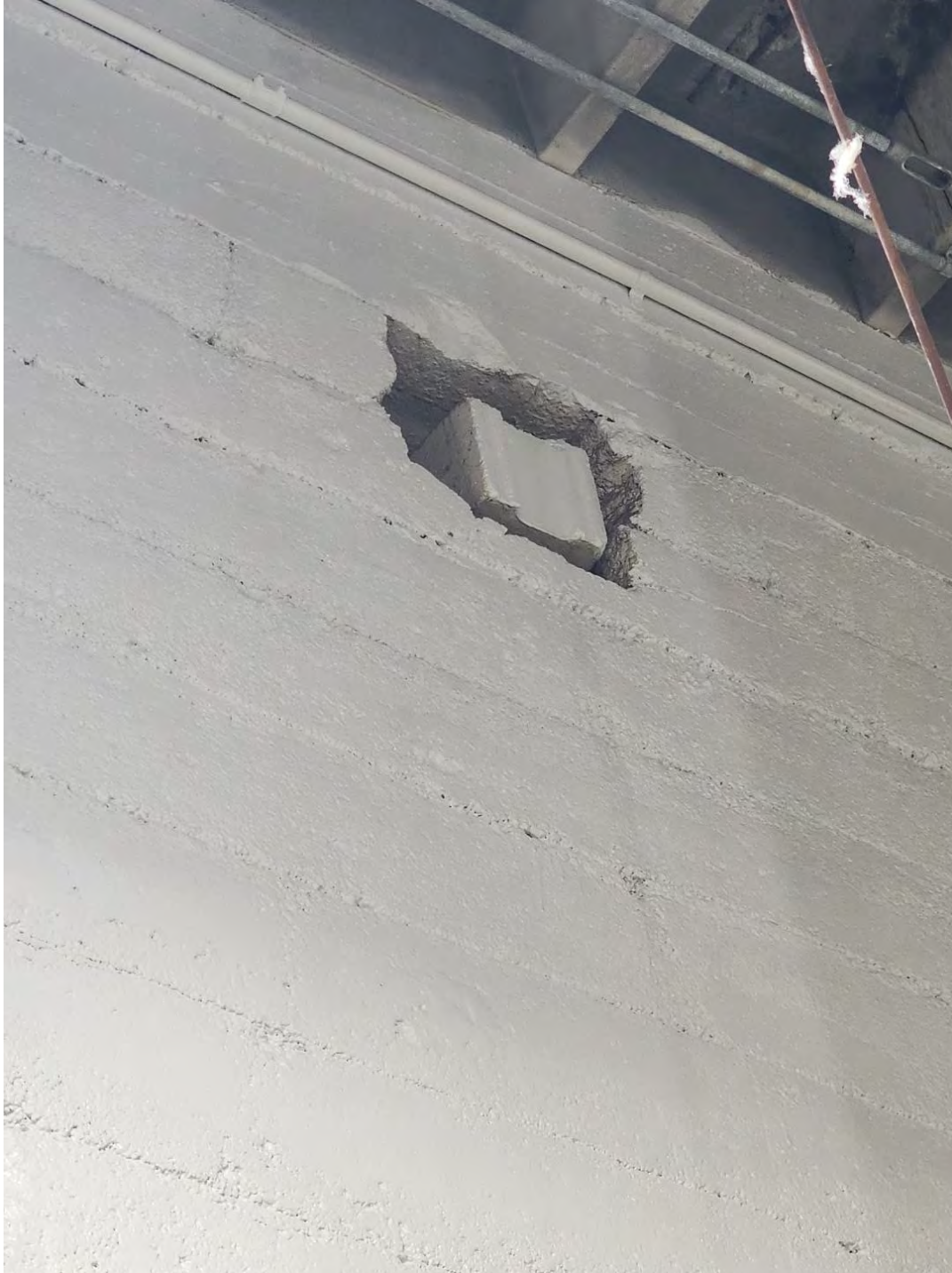
Wall penetrations infilled with non-standard construction methods. Non-rated ceiling assembly as required by building code. Location of water and pest infiltration. (Photo: 20240411_135834)
