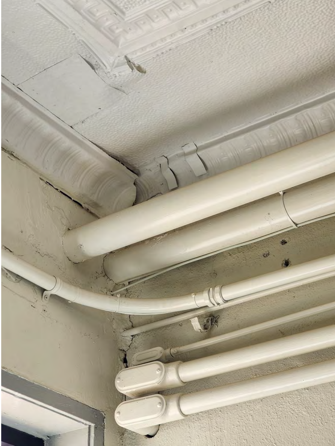
Wall penetrations not sealed. Finish material failure. (Photo: 20240411_145007)
