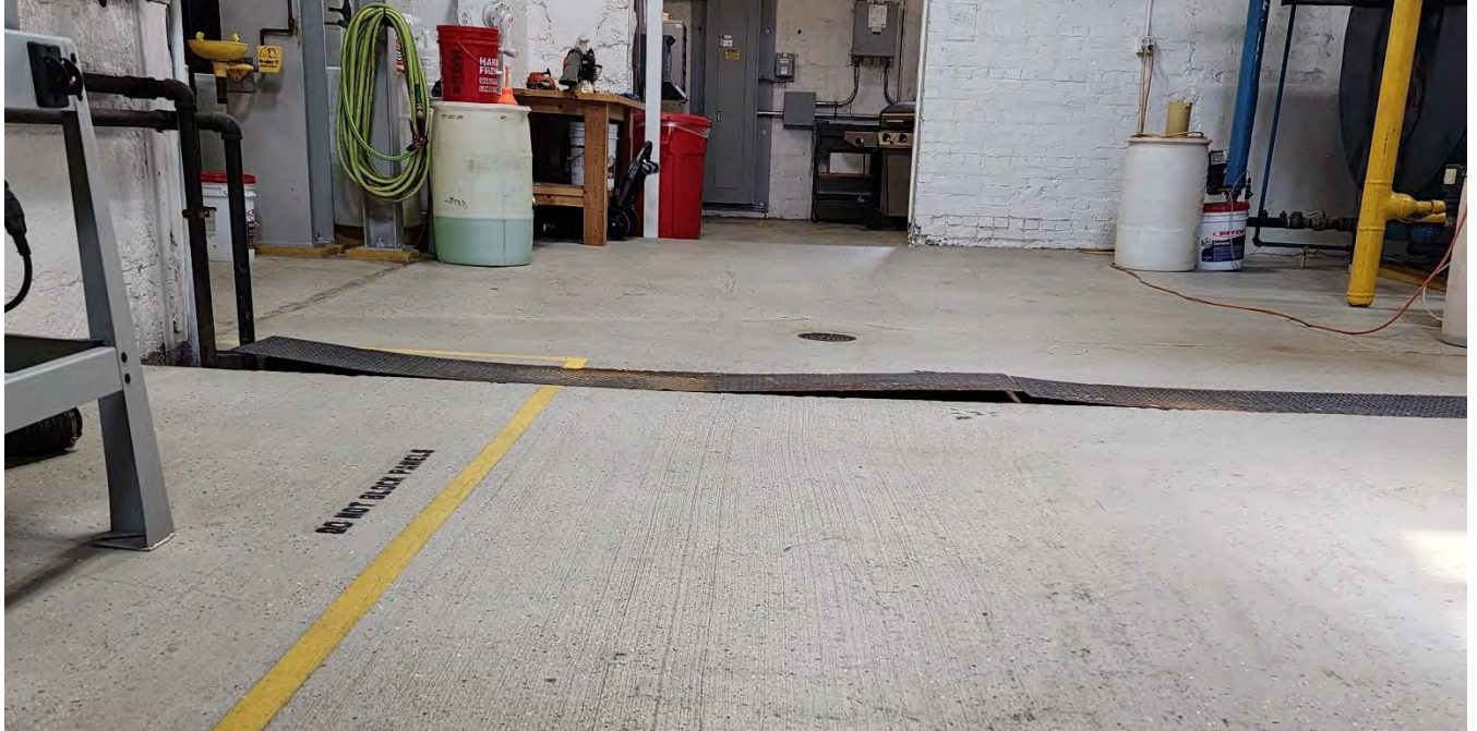
Bent trench drain covers within interior floor slab – potential tripping hazards. (Photo: 20240411_141837)
