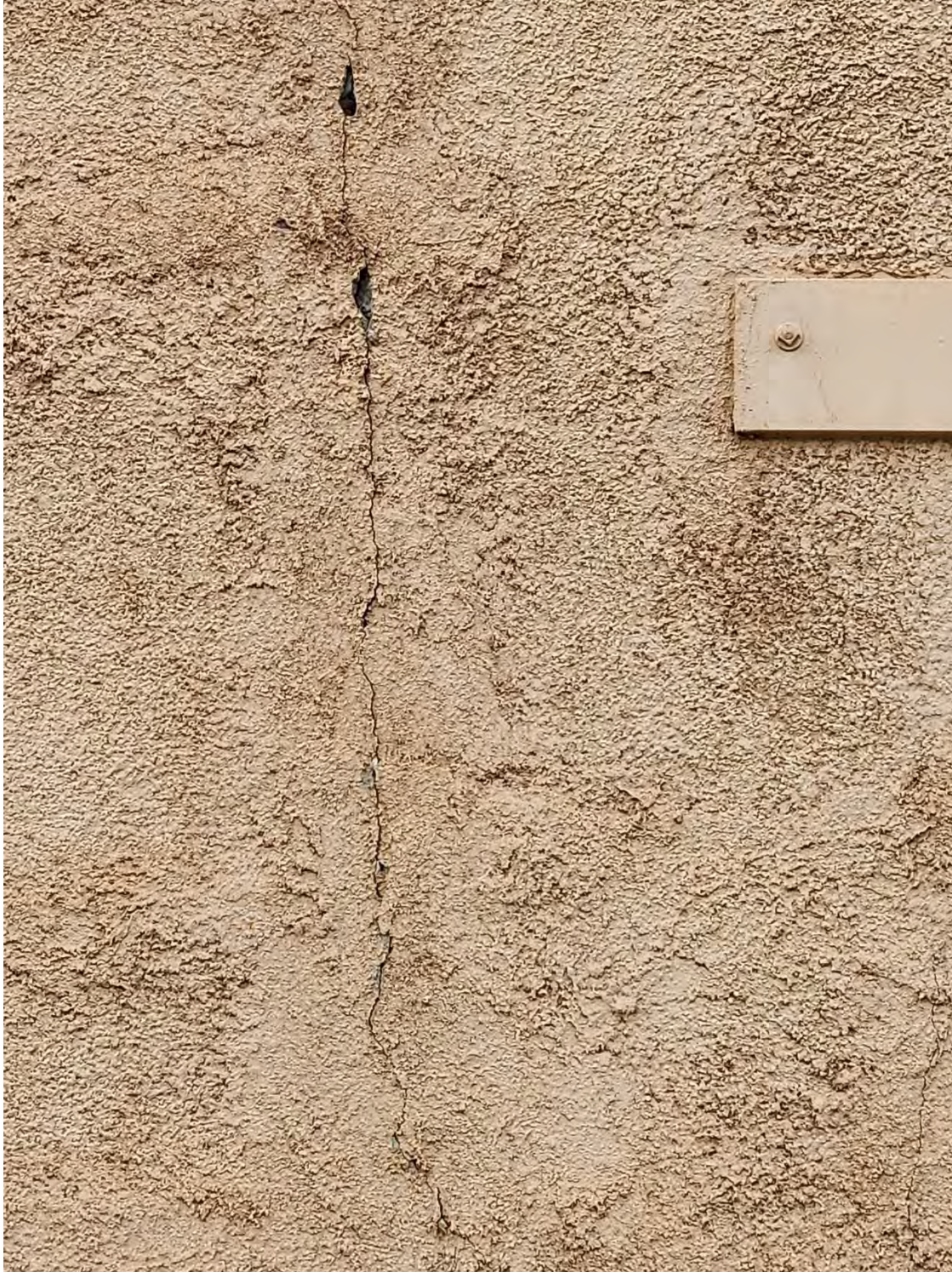
Exterior EIFS in poor condition. Extensive cracking and evidence of water infiltration causing material failure. (Photo: 20240216_143856)
