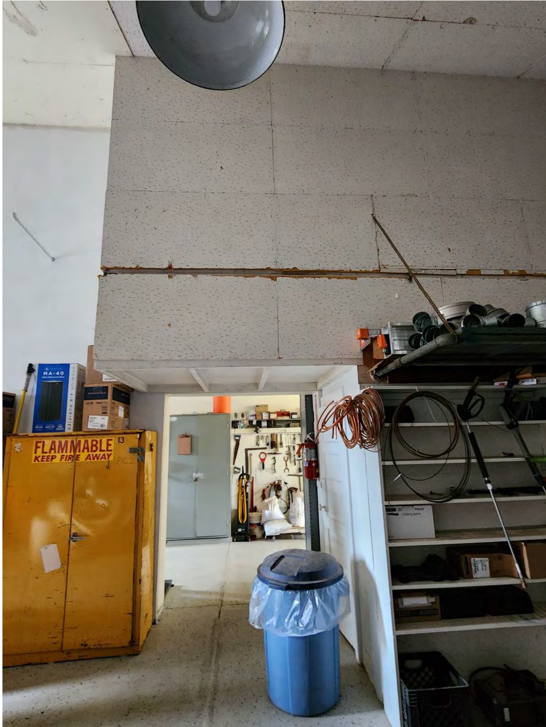
Minimum head clearance not met under stair. (Photo: 20240216_142452)
