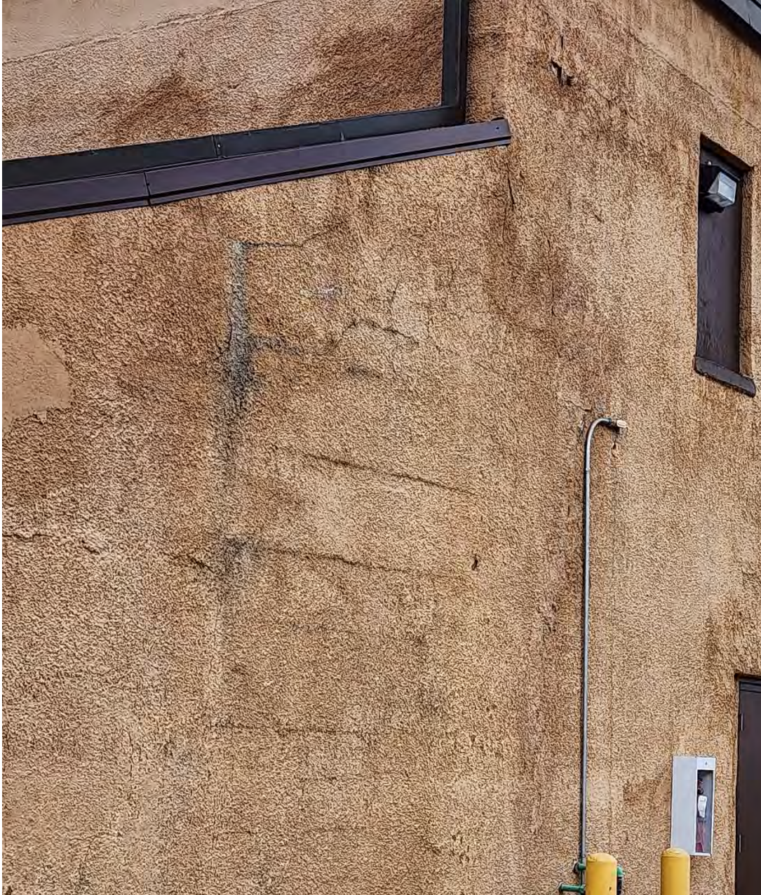
Exterior EIFS in poor condition. Extensive cracking and evidence of water infiltration causing material failure. (Photo: 20240216_143818)
