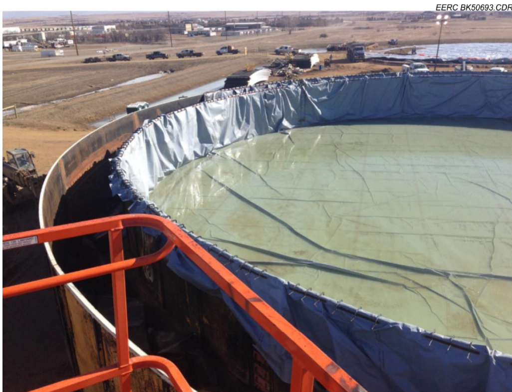
Figure 22. The double-walled water corral utilized by Statoil for produced water storage (image source: Schmidt and others, 2015).
