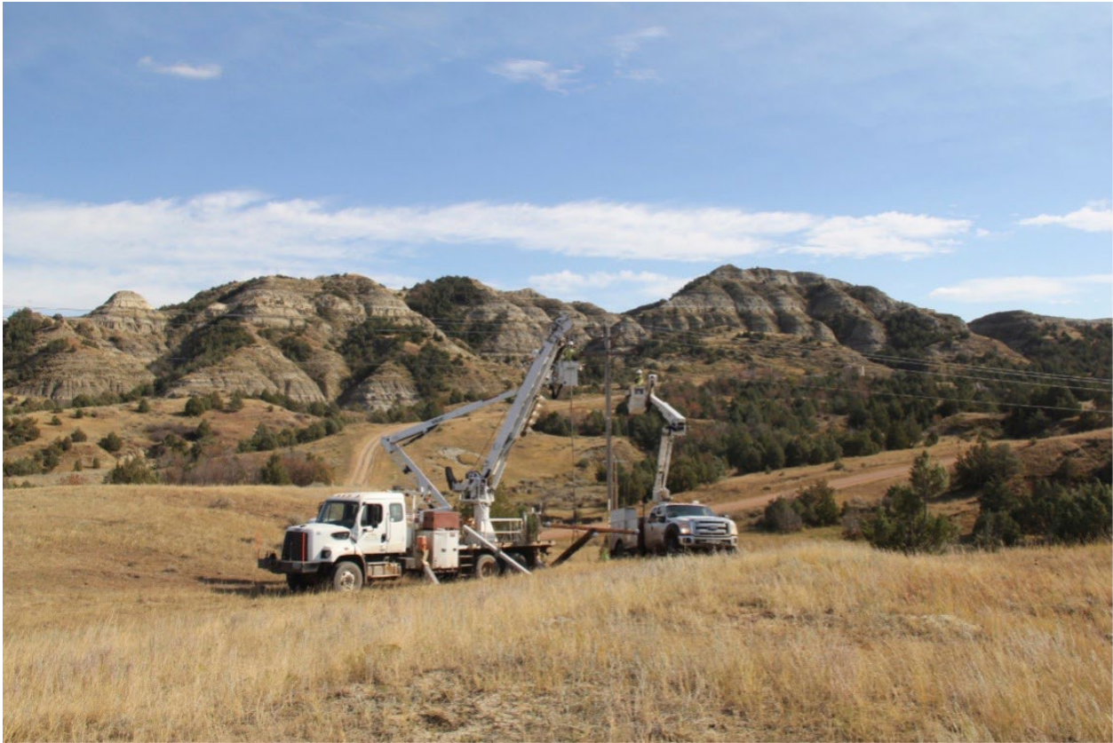
Photo courtesy Andrew Spratta – McKenzie Electric Cooperative
