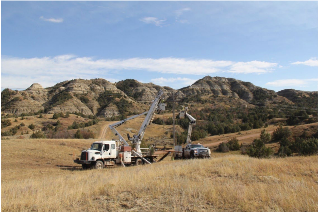
Photo courtesy Andrew Spratta – McKenzie Electric Cooperative
