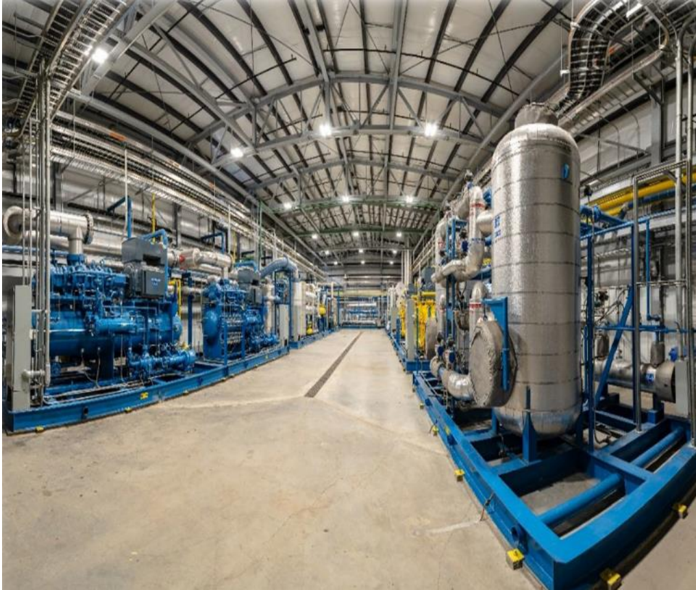
Figure 14: Photo of Completed Carbon Capture Facility
